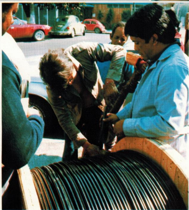
Optical fibre cable from Sieverts being installed in Mexico. The fibre optic cable offers a tremendous saving in weight and bulk. The weight of one km is about 100 kg as compared to more than 5000 kg for coaxial cable.
