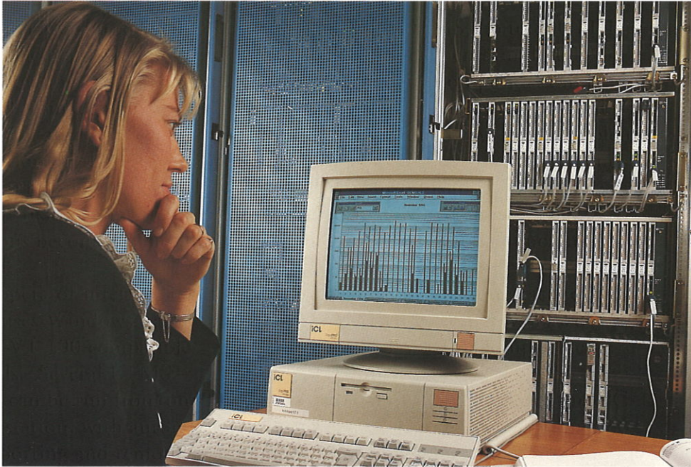
The Ericsson Transmission Management System (ETMS) collects data from PDH network elements, and presents a graphic overview of network performance.
